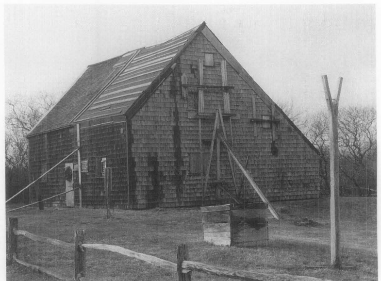
Figure 3. Buildings seriously damaged by storms or deterioration may need to be braced before architectural evaluations can be made. Jethro Coffin House. Photo: John Milner Architects.
